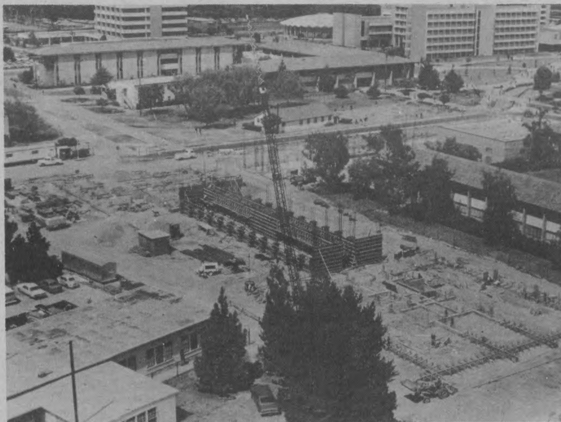
IF YOU'VE BEEN wondering what's being built, it's the South Hall Annex. Check the fence (at bottom right) for graffiti and art work.
