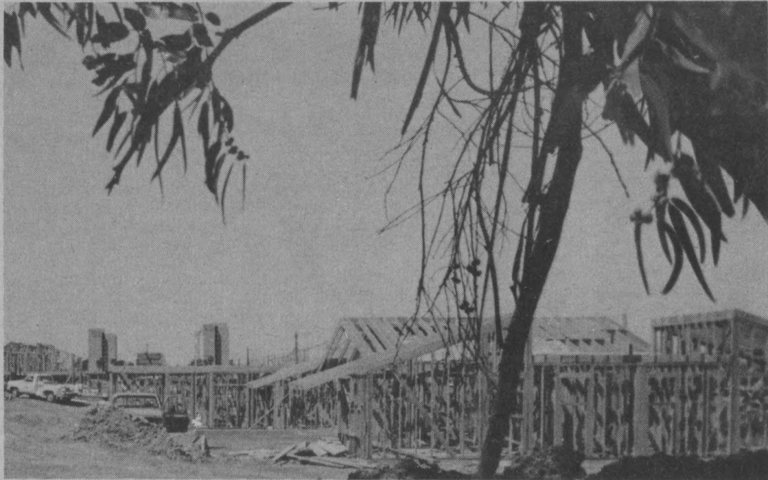
The Santa Ynez student apartments, located near El Colegio and Los Carneros, are nearing completion and will be ready for occupancy this fall.
