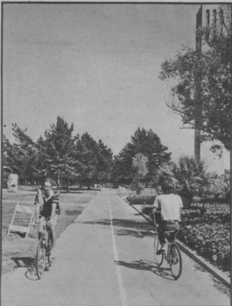
Lights are currently being installed along this bikeway behind Storke Plaza as well as the path above the lagoon. The construction is part of a plan to improve lighting on campus.
