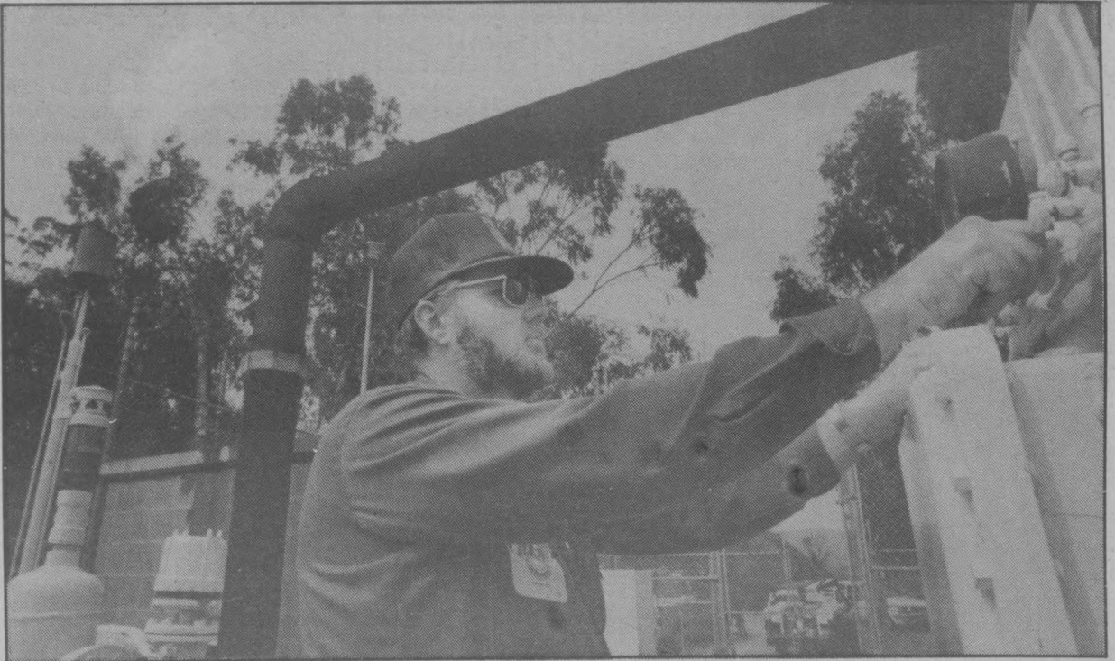
UCSB Facilities Management mechanic Walt Frowiss empties propane from pipes in a heating
