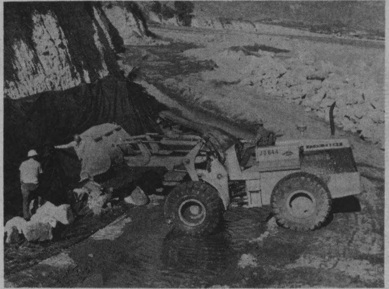
BULLDOZERS begin work on the rip-rap wall near Marine Biology lab. Construction will be finished in four weeks. Photo by Cynda Riggins
