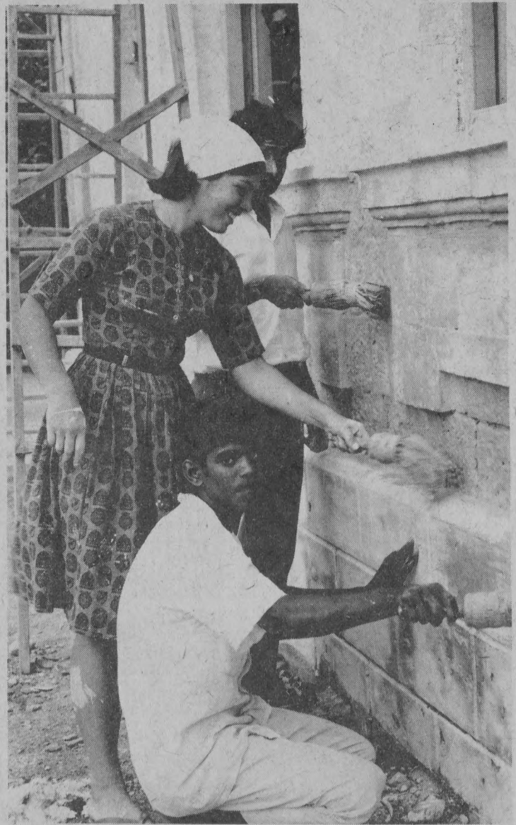
WHITE WASH THAT SCHOOL -- Cherry James, Project Pakistan returnee, works with native friends at painting a school for the blind. This was the second work project initiated by this year's traveling team from UC, Santa Barbara.
