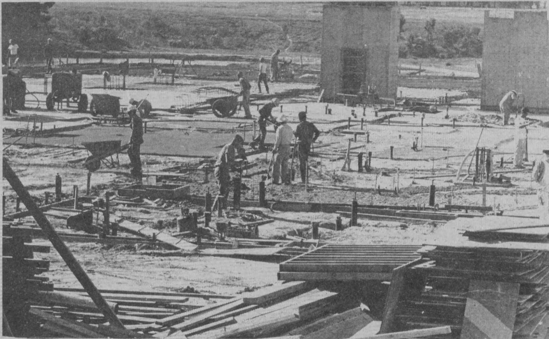
SU GOING UP -- Construction is moving onward for UCSB's new SU near the lagoon. For more on campus development see page 13. (photo by Tom Fulkerson)
