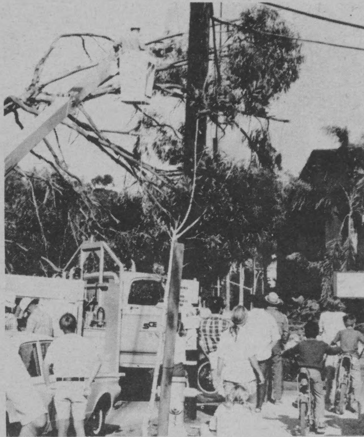
LOSE YOUR POWER SUNDAY??? If you did, the villain was this eucalyptus tree which fell on a power pole at the corner of Embarcadero Del Norte and El Colegio. But the gallant heroes of SCE restored our electricity in less than an hour.
