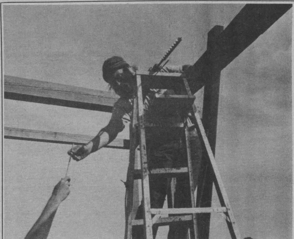
A HELPING HAND — The sign-post at Madrid Park begins to take its form as workers are kept busy with construction on the project.
