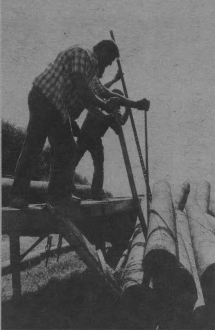
Construction on an Isla Vista Seawall to help control erosion along the Del Playa cliffs began yesterday.
