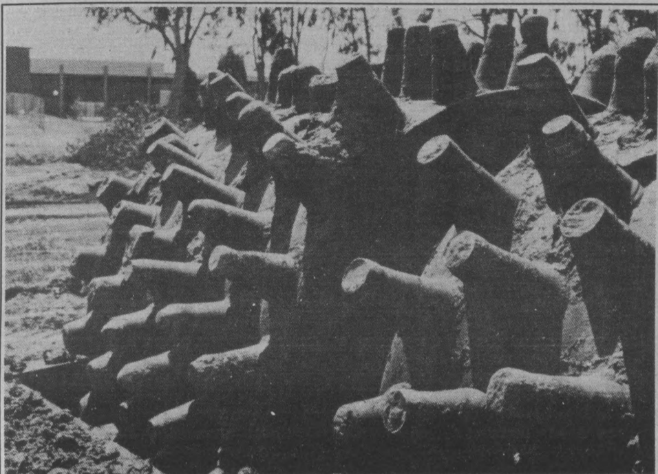
ALREADY ROLLING- Only days after a Superior Court Judge ruled in the University's favor, heavy construction equipment moved in to begin work on the Campus Events Facility. See story below. (Photo by Eric Woodbury)
