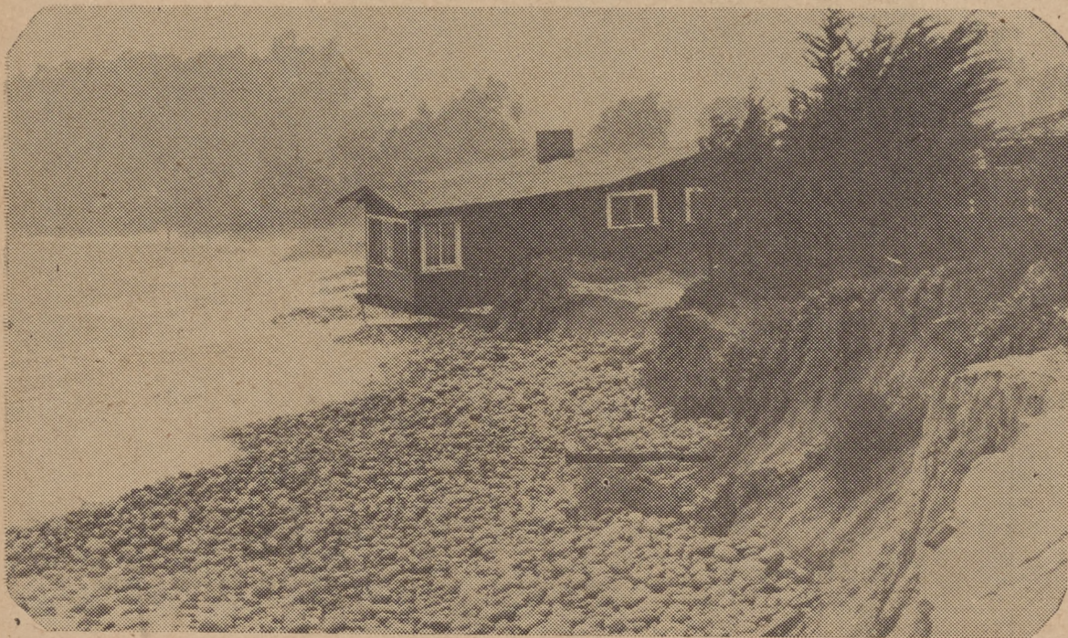
The Frank Nagle beach house in Serena which was the first cottage to fall prey to encroaching seas. Picture courtesy News-Press.
