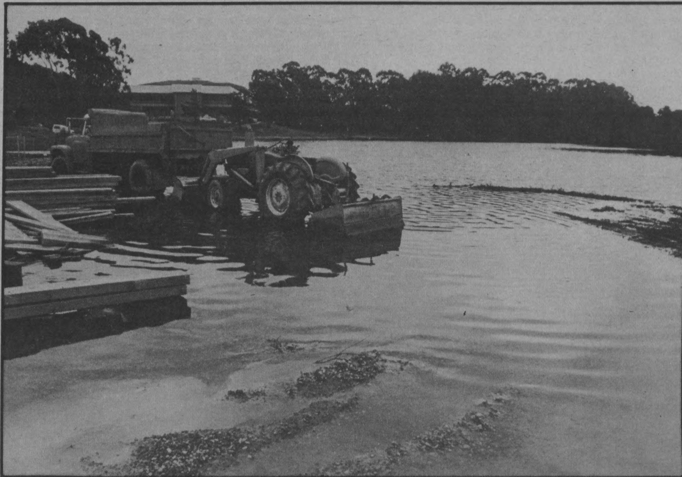
Campus Swamp — Heavy rainfall expanded the lagoon over the weekend, forcing construction crews to temporarily abandon their equipment. See story on page 3.
