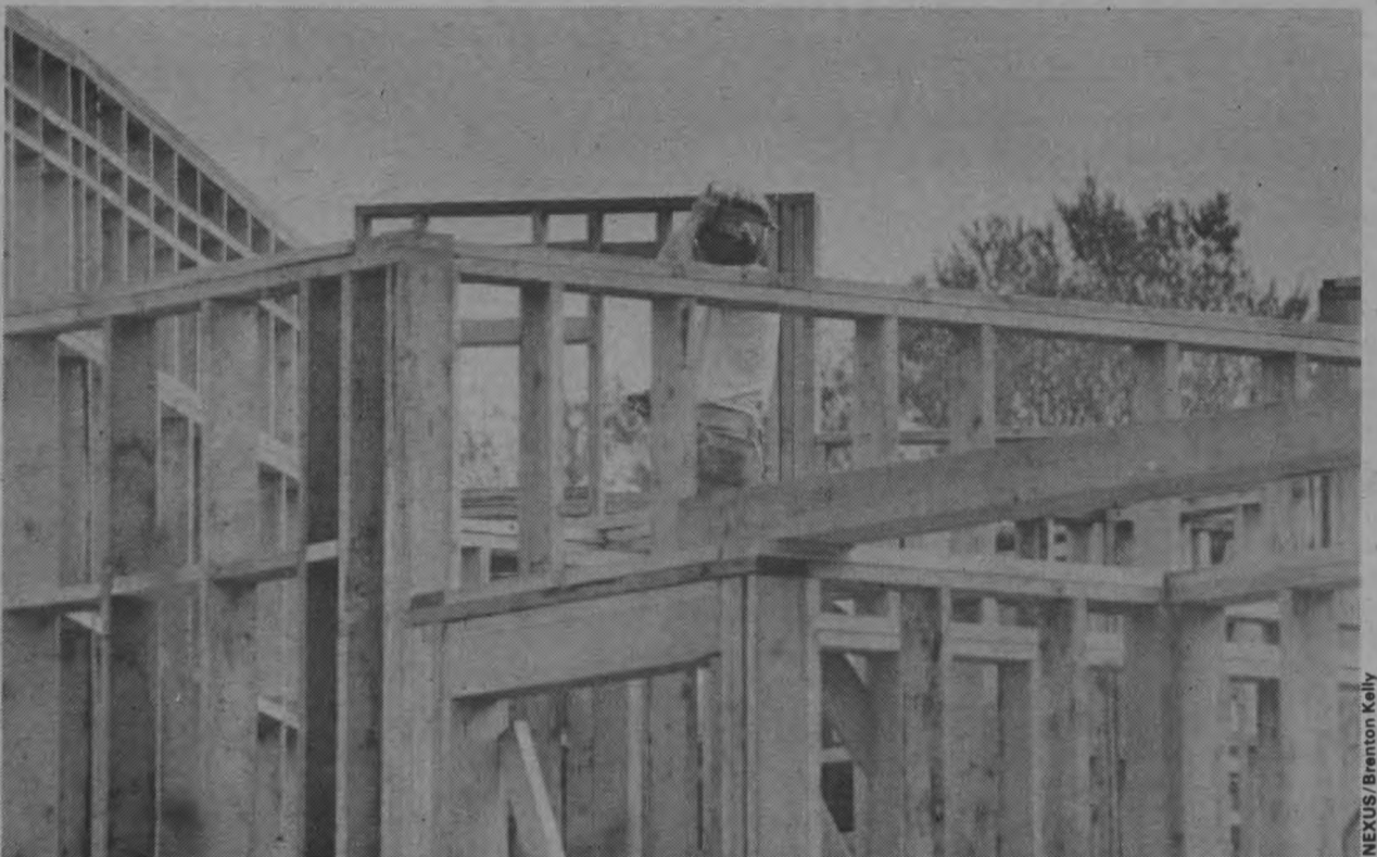
A construction worker on the new Student Services Building at UCSB pauses in the mid-day heat.
