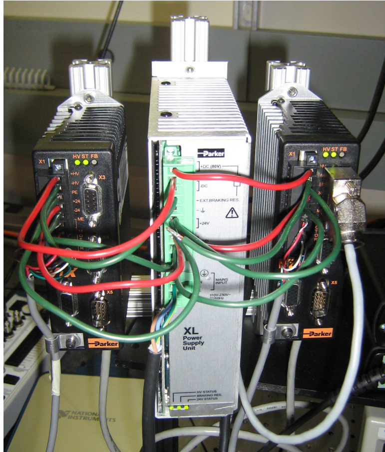
Figure A.8: Driving the two stepper motors are three pieces of Parker electronics: in the center is a power supply which powers the controllers on the left and right.
