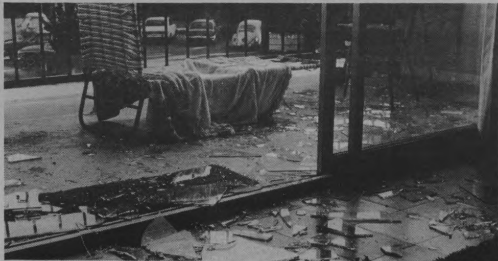
Damage like this to a Del Playa apartment occurred Aug. 13, 1978 during an earthquake registering 5.6 on the Richter scale. Today, UCSB buildings face ongoing checks in an effort to make the structures safe during a future earthquake.
