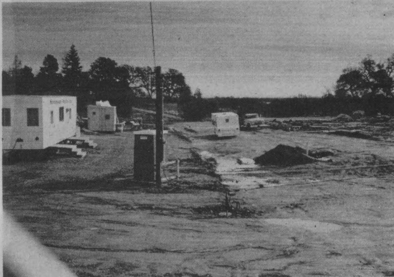
On this site approximately 10 miles east of Sacramento, the new Governor's mansion is rising.
