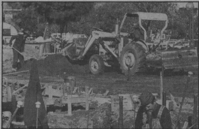
Workers lay the foundation for the Biological Sciences building which will be completed by August 1985.
