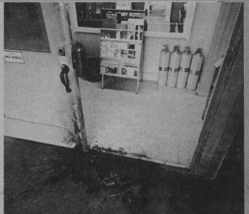
BOMB DAMAGE to entrance of ROTC building. The FBI is investigating
