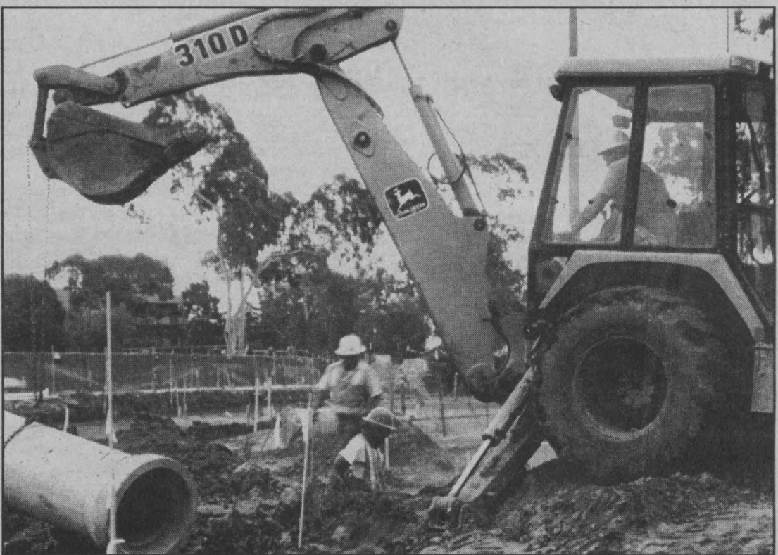
Bulldozers work diligently to construct the new parking garage, which is expected to be complete by the end of the year.
