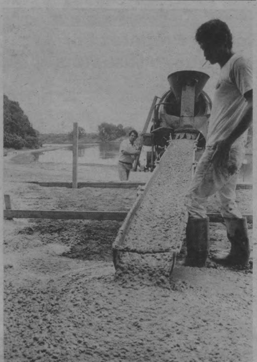
Workers pour cement outside UCen where picnic tables will soon be located.
