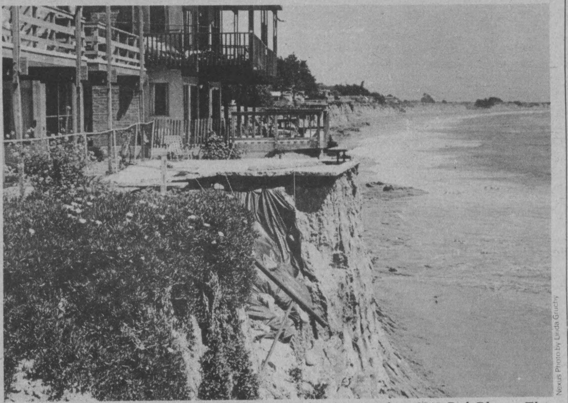
A plastic tarp covers the area where a porch once stood at 6745 Del Playa. The occupants fear further erosion of the bluff.
