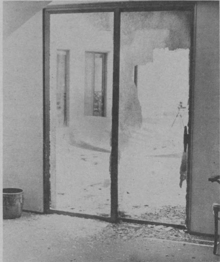
THE FORCE OF THE BLAST blew Dover O. Sharp from a position directly to the right of this shattered door back 15 to 20 feet. Pieces of charred clothing and dried blood mark where he landed.
