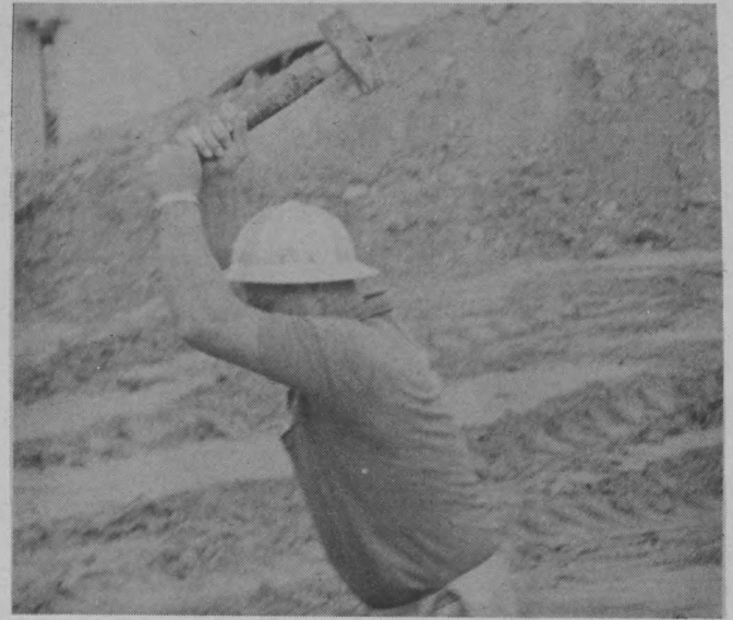
THOR STRIKES AGAIN!?! No, it's not even someone who feels bad because his girlfriend told him to go pound salt; he is one of the construction workers that keep the Storke Communication Building going up ahead of schedule. —photo by Chuck Markham
