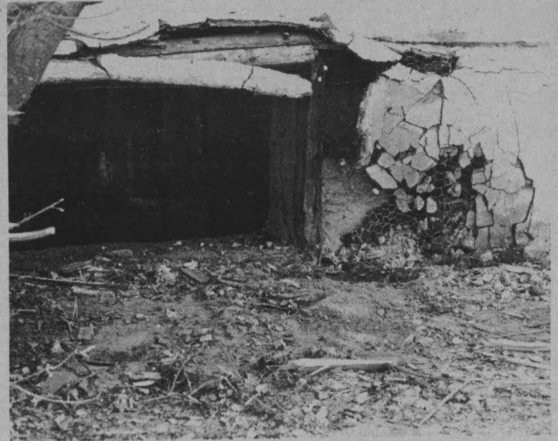
A BOMBED-OUT VENT in the Santa Barbara National Guard Armory.
