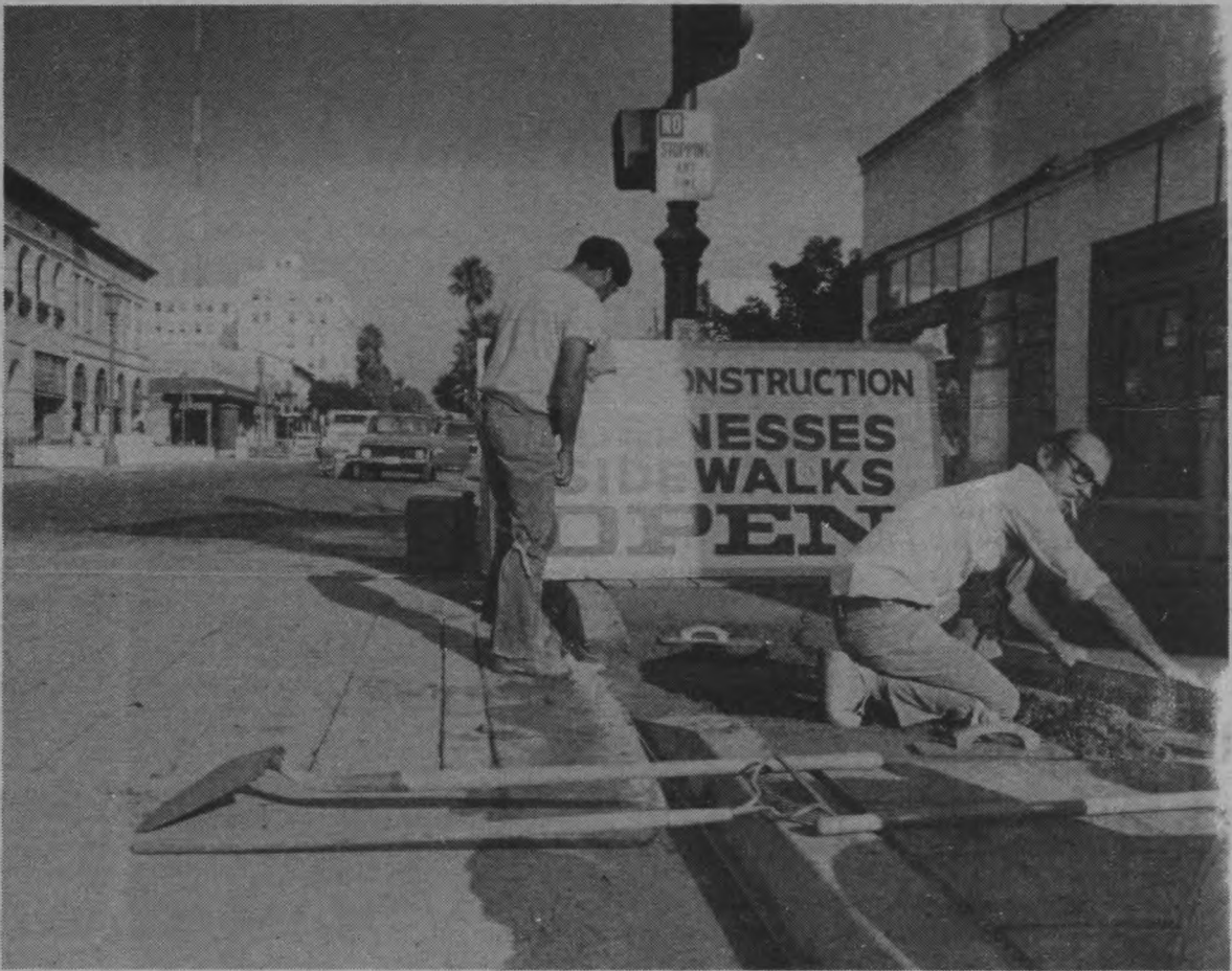
City workmen labor to finish downtown reconstruction of lower State Street. The block is scheduled to be completed Oct. 15.
