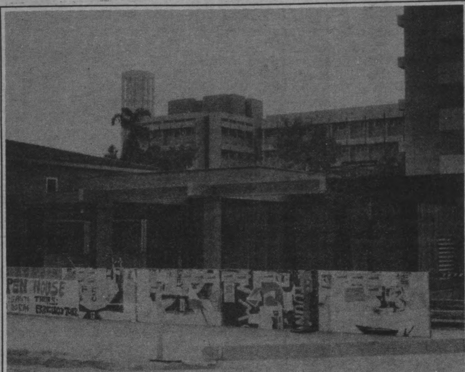
LIBRARY EATERY — Now under construction, this new snack bar by South Hall will hopefully satiate any red-eyed, starving student who finds the lines at the UCen or Ellison snack bar too difficult to negotiate.
