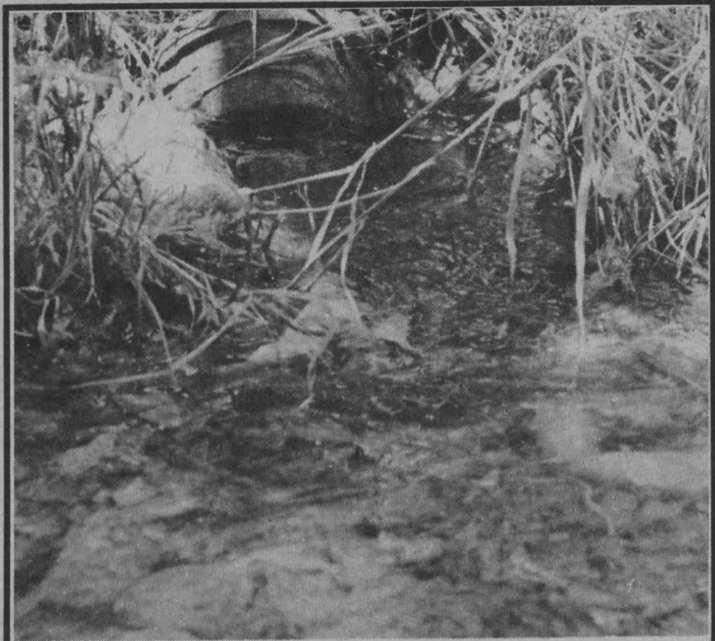
Raw sewage leaking from a plugged up sewage pipe caused this scene on 777 Embarcadero del Mar.
