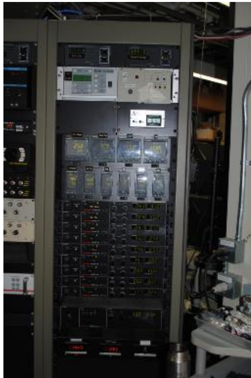
Figure 8 -- Right side of the Nitride Gen II electronics cabinet.
